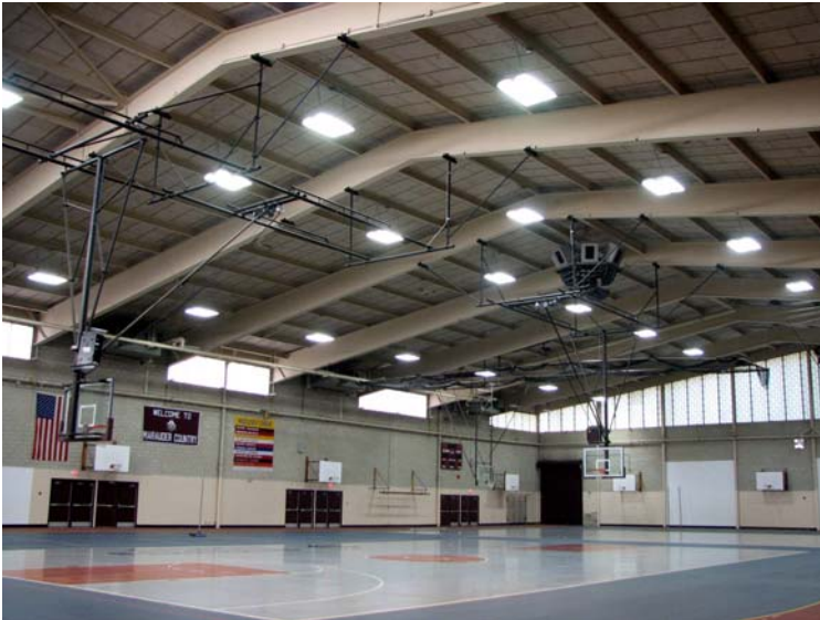
Energy efficient lighting in use at the Belmont High School field house
